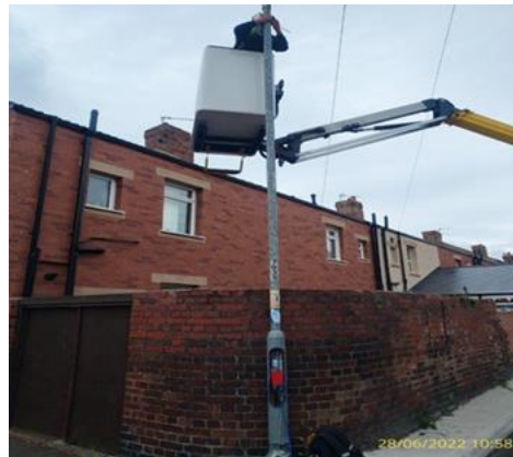
CCTV attached to lighting column
