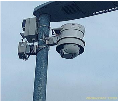
Close up of CCTV unit
