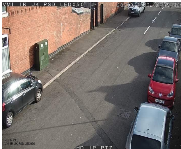
(hotspot after CCTV installation)
